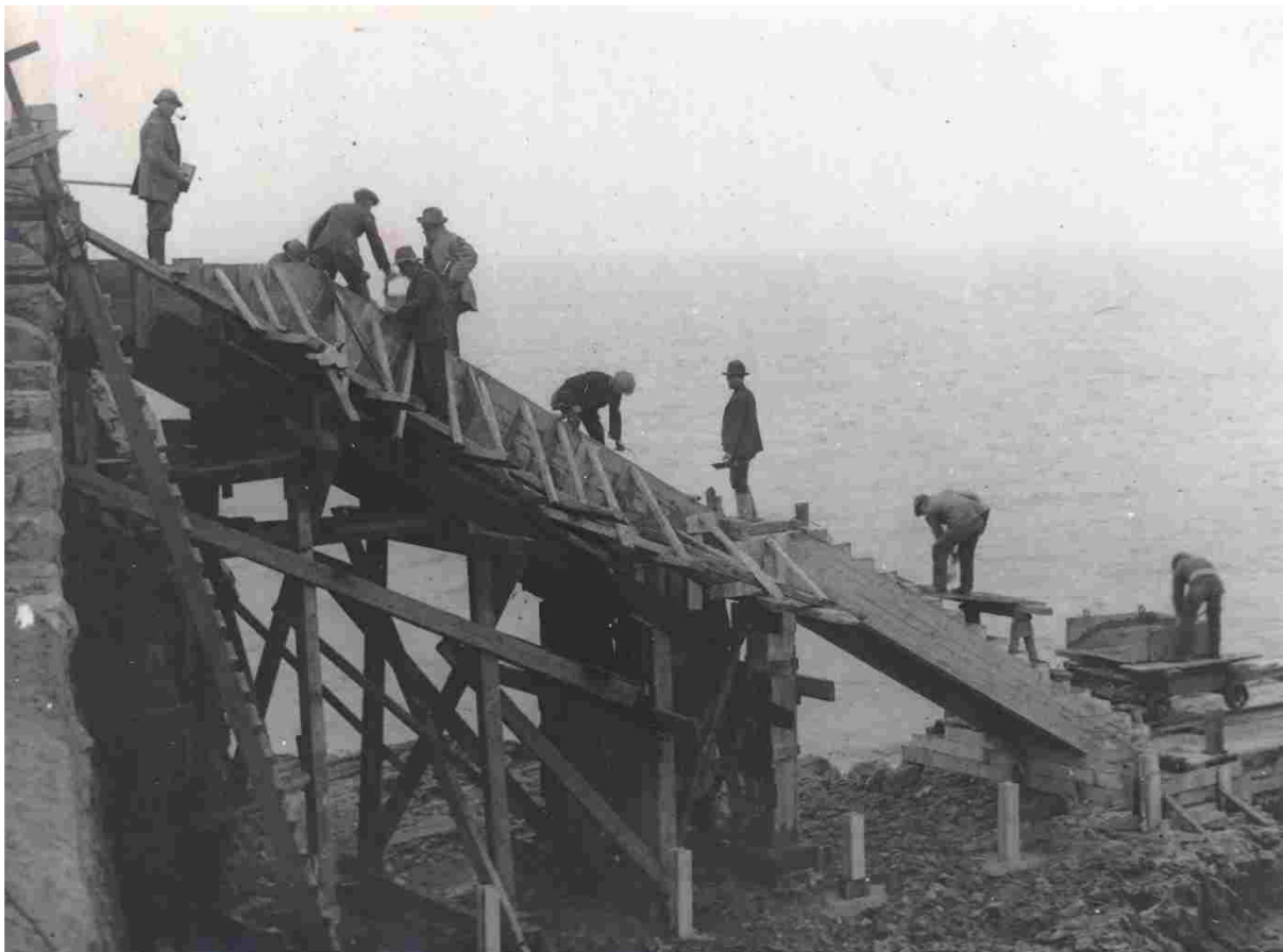
Work begins to connect Knightstone Island to the site of the new causeway
